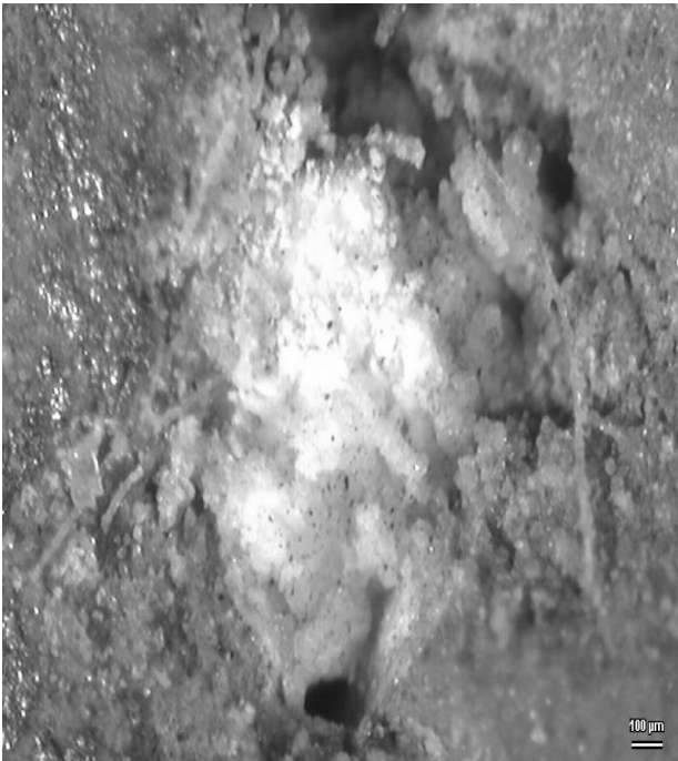
Figure 7. An extensive lime nodule observed on the surface of the sample No. 1 - old technology fired roof tile.
